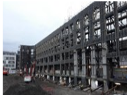
Internal view of the facade retention and propping along the Queensway elevation
